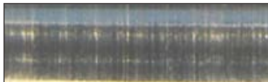
Condition at depth of around 100mm
